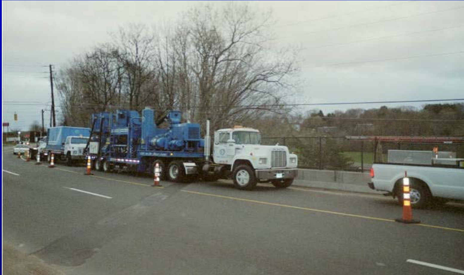
Equipment train, abrasive recycling equipment
