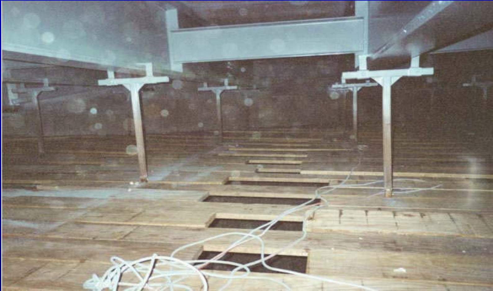
Traditional containment on hangers
