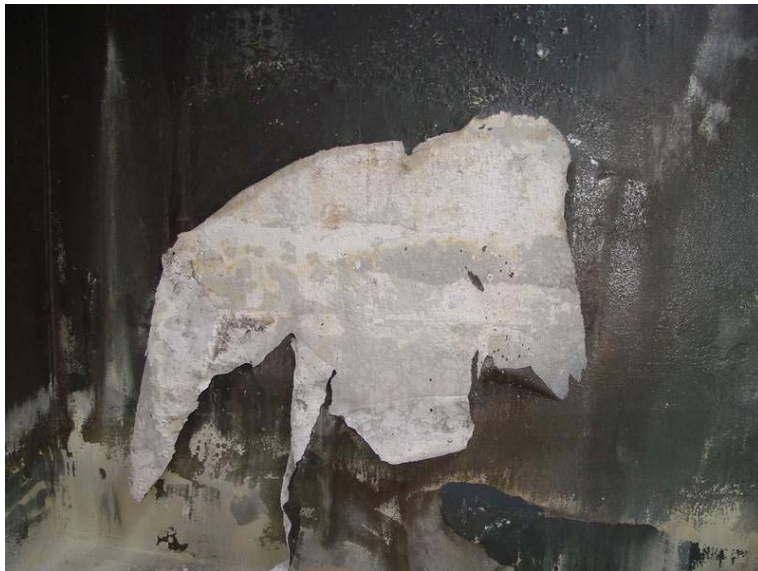
Figure 7: Lift Station failure
