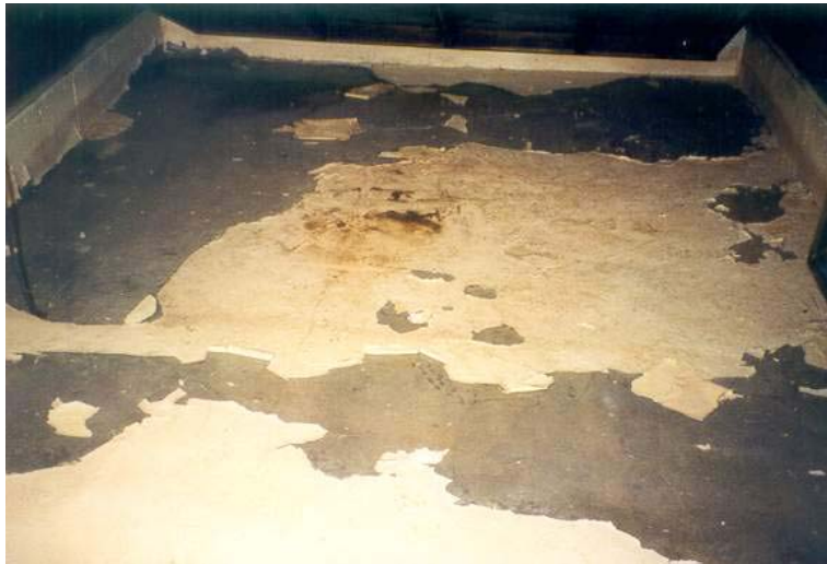
Figure 3: Disbonding of the polyurea system
