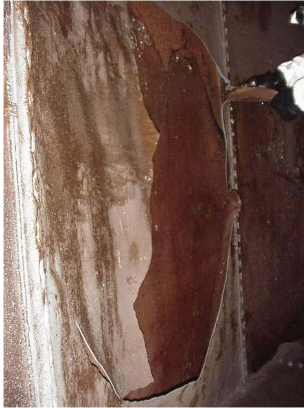
Figure 5: Wastewater tank lining failure
