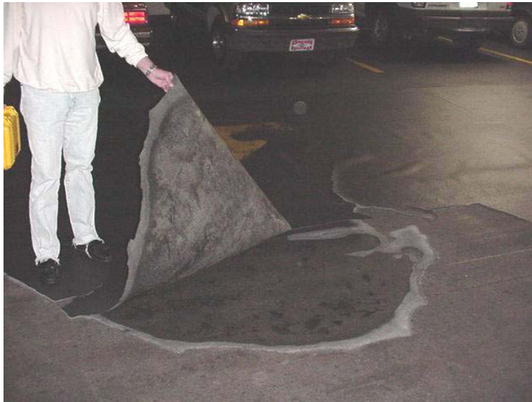
Figure 6: Casino Parking Garage Failure
