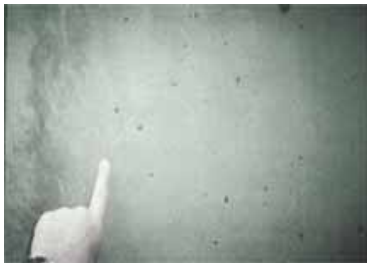
One of the problems with mass cast, steel-formed concrete is surface “bugholes” and voids.
